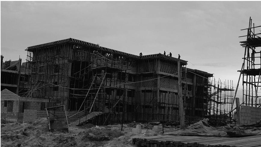
Photo 8.2 Dar es Salaam. A picture showing a group of informal construction workers working at height without any form of PPE while the site housekeeping is not well arranged.
