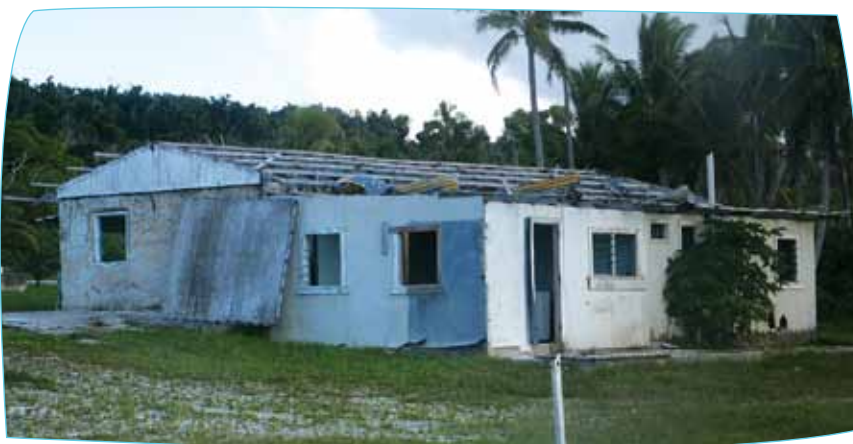
House damaged by Tropical Cyclone Heta, January 2004.
