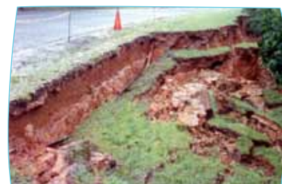
Landslide during Tropical Storm Utor in June 2001.
