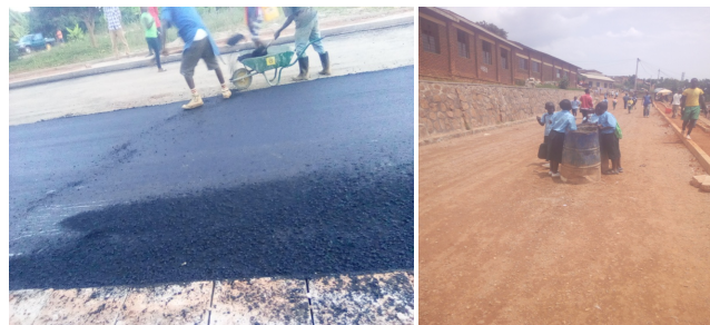
Figure 2. Lack of safety measures to road Workers for asphalt and land surveying activities and road users like children.
