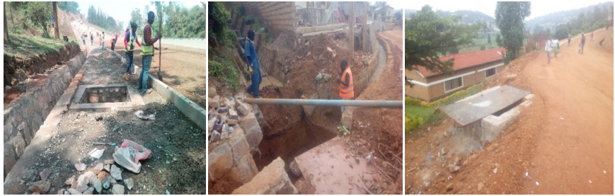
Figure 10. Lack of protective information for Manholes at Karama, Akagera and Agatare roads respectively.
