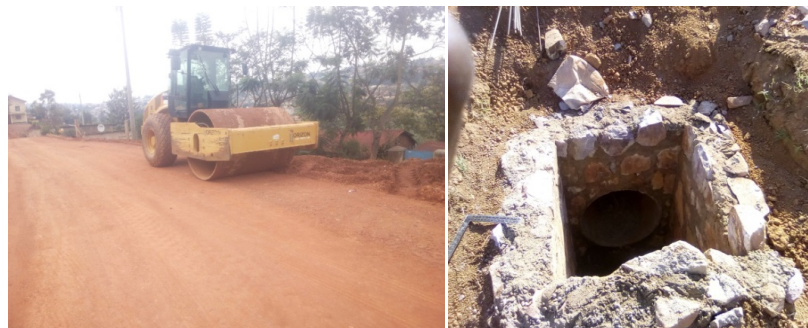
Figure 12. Lack of Adequate Signs to warn parked Machine at Karama Road and a manhole under construction at Akagera Road.
