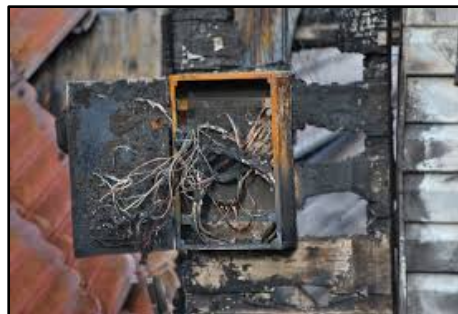
Figure 12. External main board fire.
