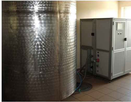
Figure 1. Industrial system for an incorporating stochastic noise water softener.
