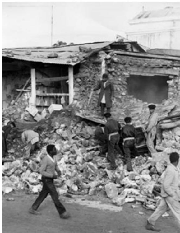
Figure 4. An example of damage to a rubble stone and mud house. Photo from Sulfium Forum [21].
