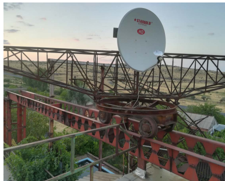
Figure 5. Ku-band, 100 cm dish antenna and LNB of ArtAr-HDF are installed on mechanical scanner at a height of 10 m from the ground in experimental site of ECOSERV ROC Co. Ltd. near the Village of Ujan and directed West to measure sky emission and solar emission during sunset.
